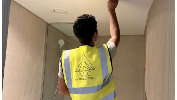
DAMAC LAGOONS / DUBAI — RECTIFICATION DETAIL
